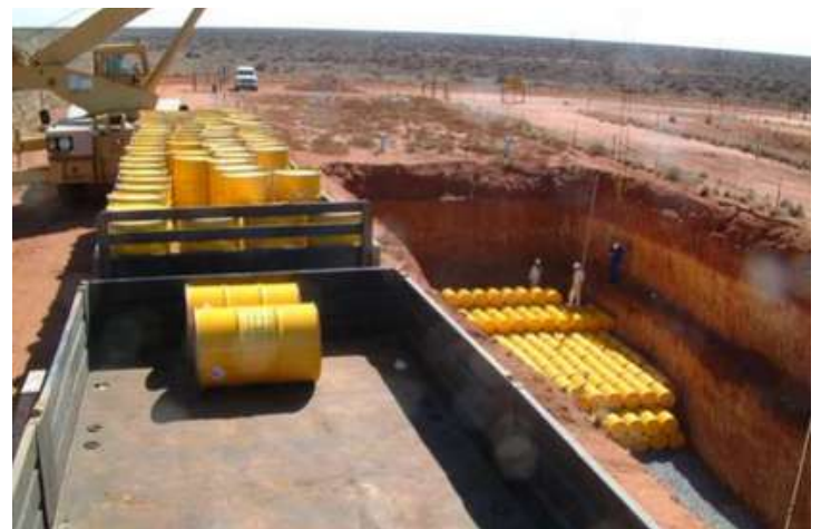
LLW metal containers being emplaced in a disposal trench - Vaalputs National Radioactive Waste Disposal Facility Public Information Document (PID)
